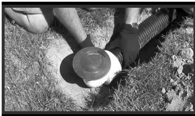
Pop Up Drain Valve Termination
