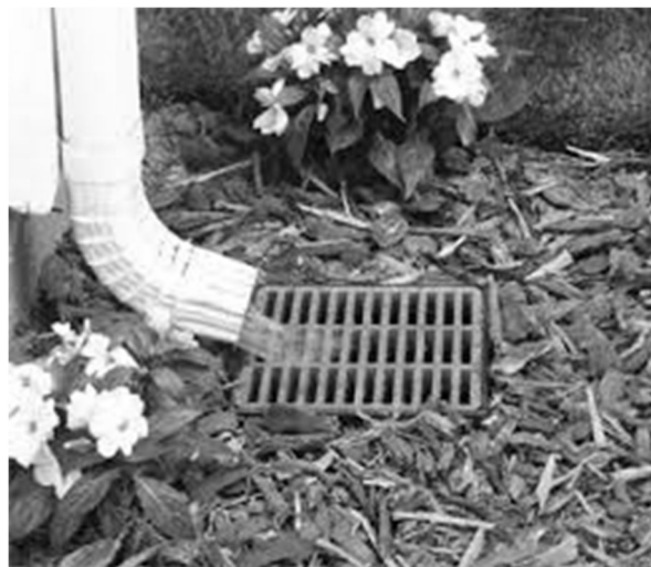
Inlet Box with a Grate
